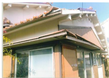
庇の腐朽・破損
